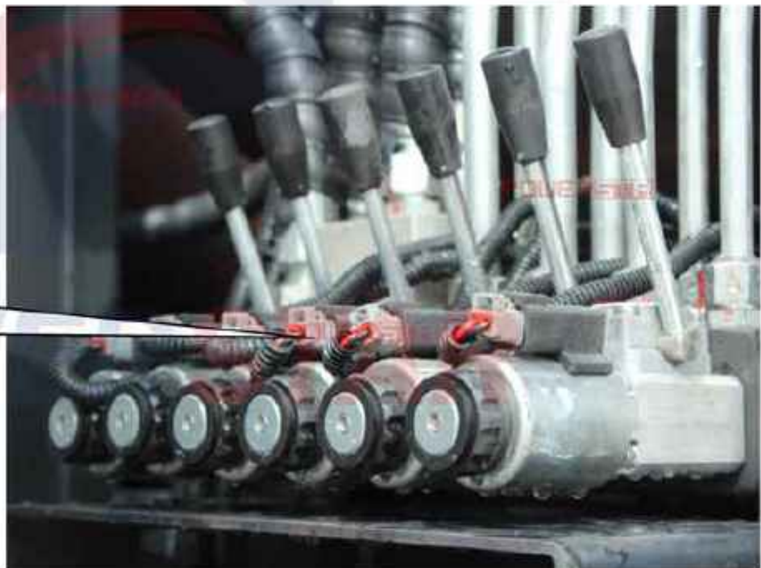
Hydraulic Control Joysticks (At drive side)
